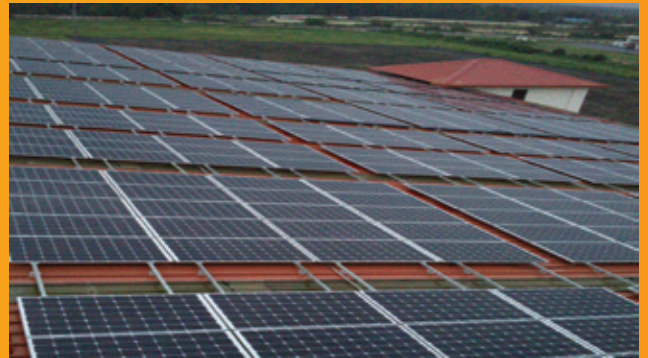
CIAL, KERALA - 1 MW p SLOPED SHEET ROOF
