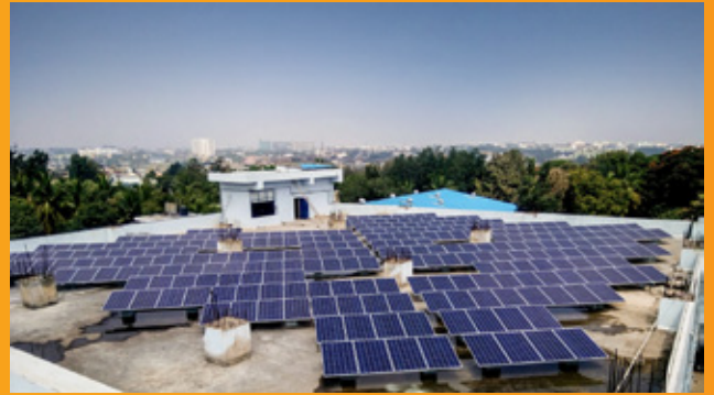
MIDC, MUMBAI, MAHARASHTRA - 200kW p FLAT RCC ROOF
