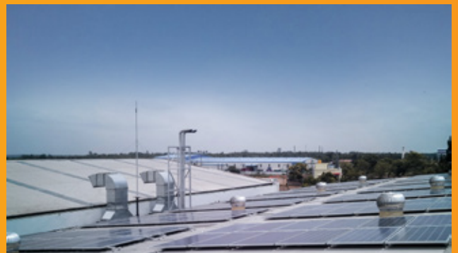
CATER PILLAR, HOSUR, TAMILNADU- 150 kW p SLOPED SHEET ROOF
