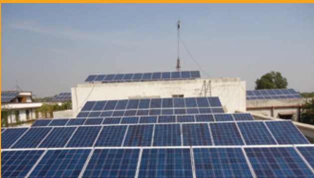
GANDHIDHAM, GUJARAT - 300 kW p FLAT RCC ROOF
